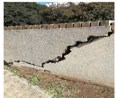
Cracked wall outside OT workshop
