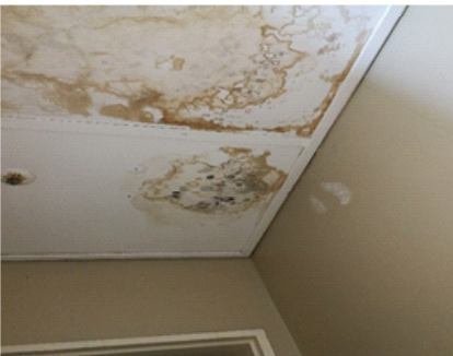
Ceiling damaged from leaking roof
