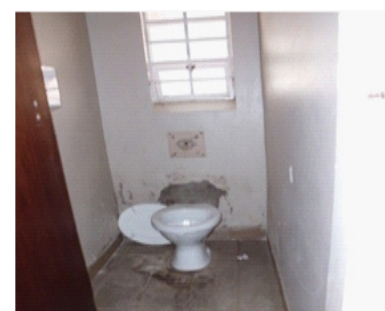
Broken Toilet in OT Department
